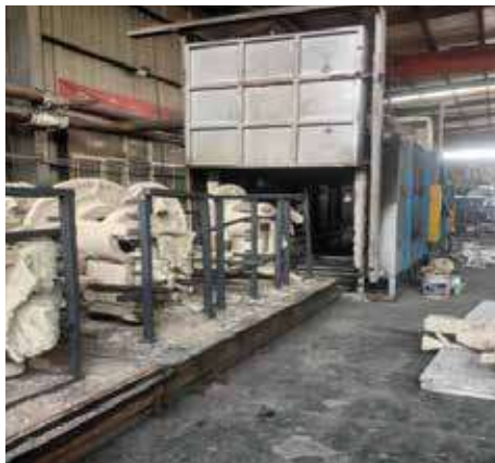
High temperature roasting furnace in shell lost foam casting
